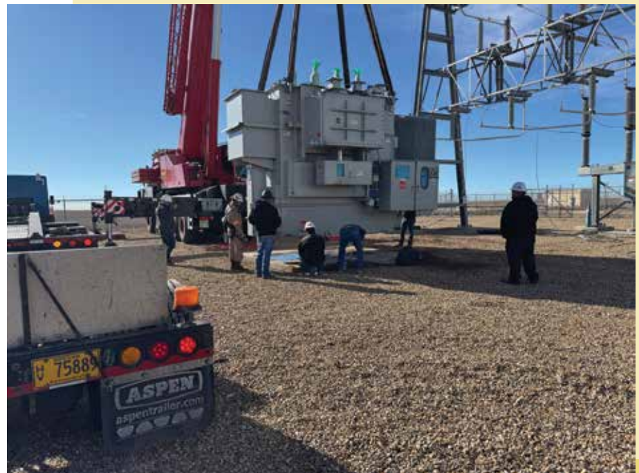
Shown here, Rita Blanca Electric Cooperative replaces a transformer in the Spurlock/Flyer Substation. Rita Blanca was a recipient of federal funding through the U.S. Department of Energy's Grid Resilience and Innovation Partnerships program to construct approximately 55 miles of new transmission near Dalhart, Texas. This is one of many examples of Golden Spread Members working to secure grant funding that strengthens infrastructure in the region.
